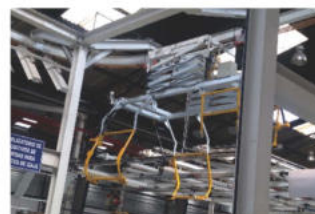
Over Head Conveyor System
