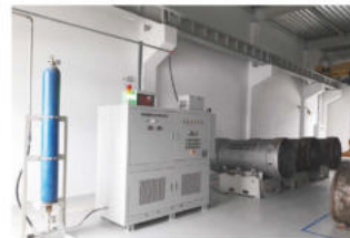
Refrigerant Outside Supply Equipment
