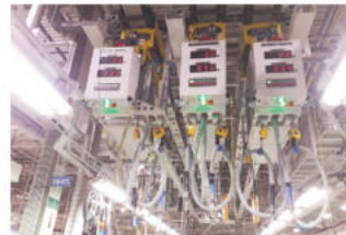
Refrigerant Charging Equipment
