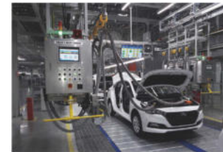
Coolant Filling Equipment
