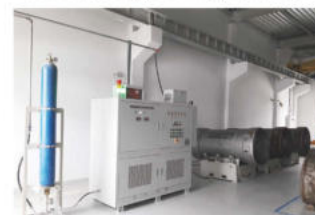
Refrigerant Outside Supply Equipment
