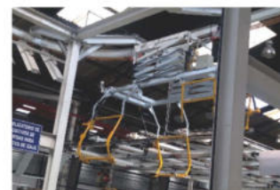
Over Head Conveyor System
